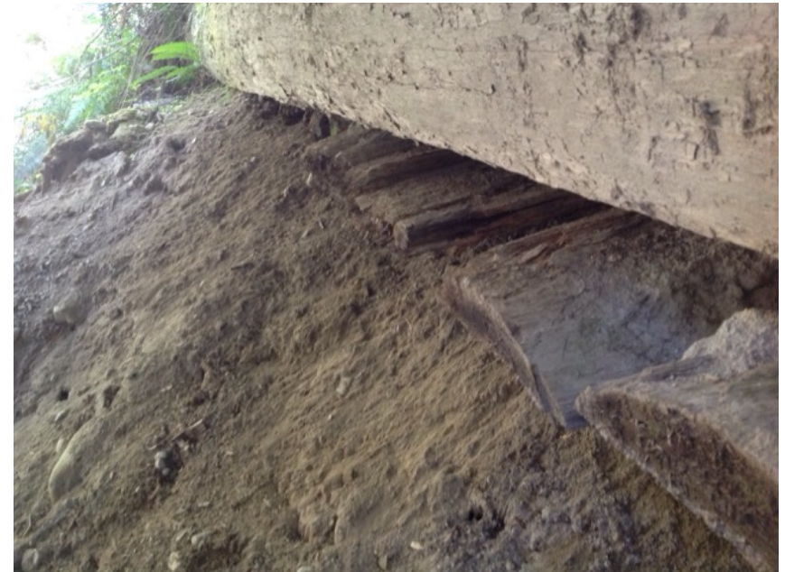
log retaining fill of left bank in front of log sill scoured
